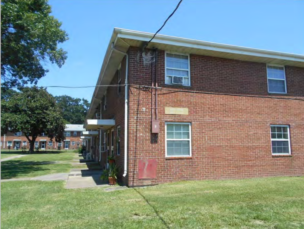
Overhead electrical lines within close proximity of the windows
