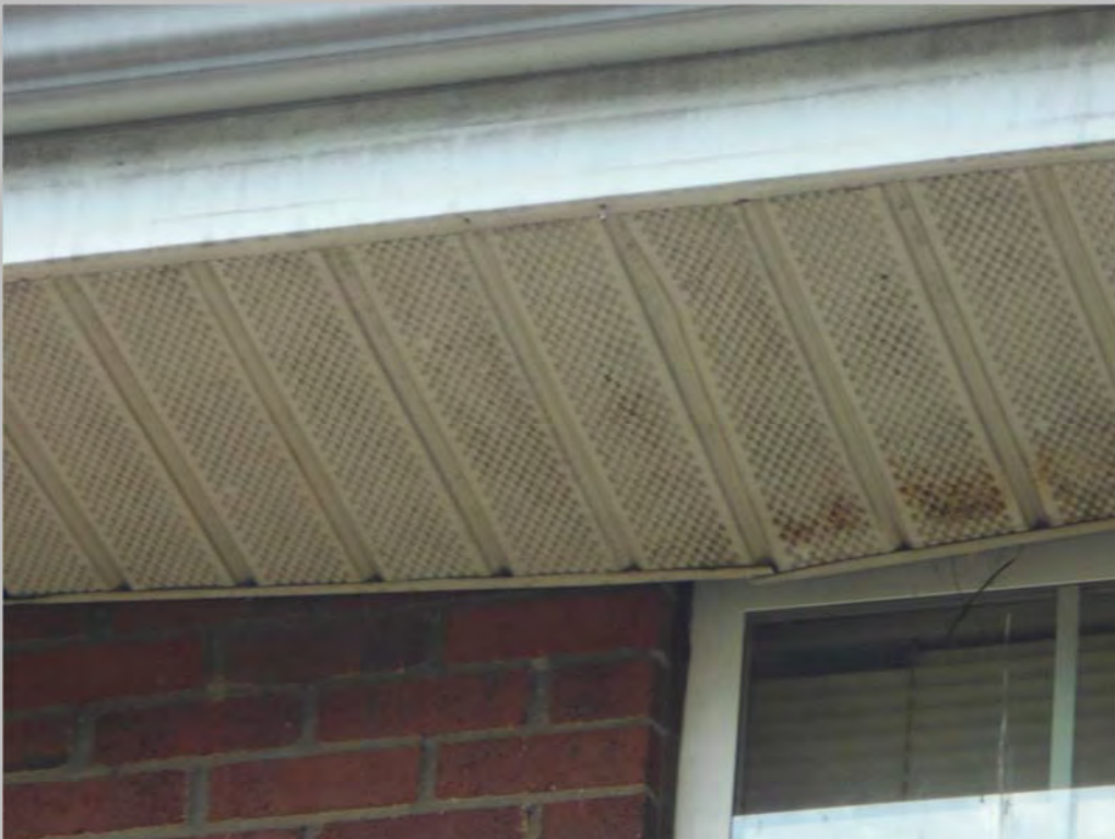
Typical deteriorated soffits
