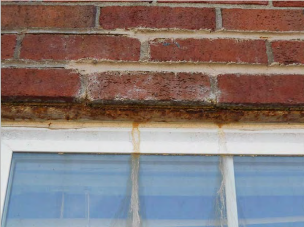
Typical deteriorated steel lintels
