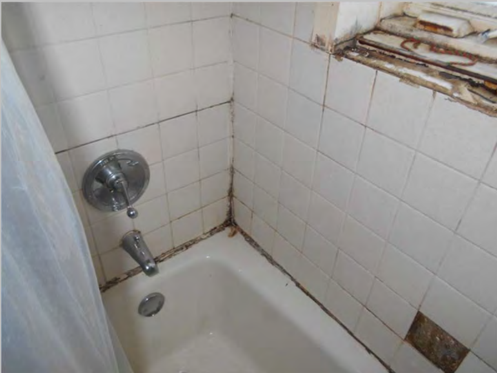
Typical dwelling unit bath tub and ceramic tile surround
