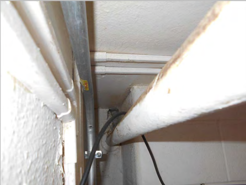
Surface-mounted piping and raceways typical in all dwelling units
