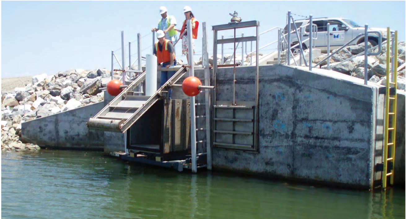
Figure 2-6: Example of a tide gate (downstream side). As water level rises, buoyancy forces act on the orange floats to shut the door.
