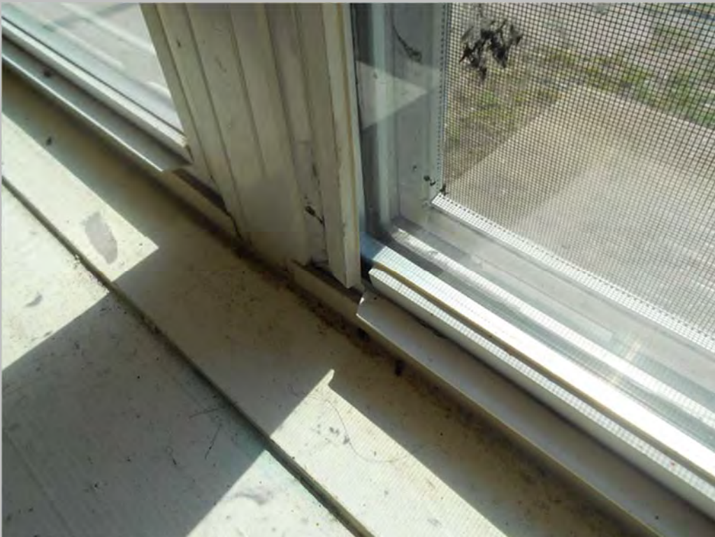
Typical dwelling unit windows – damaged and poorly installed
