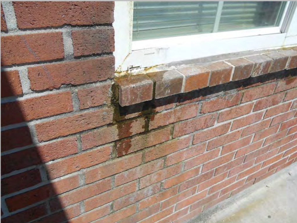
Typical deteriorated and stained brick masonry
