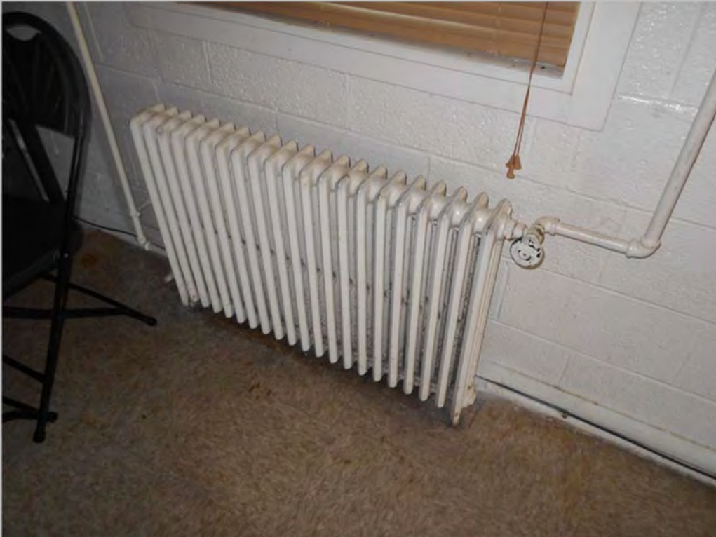
Typical dwelling unit hydronic radiator
