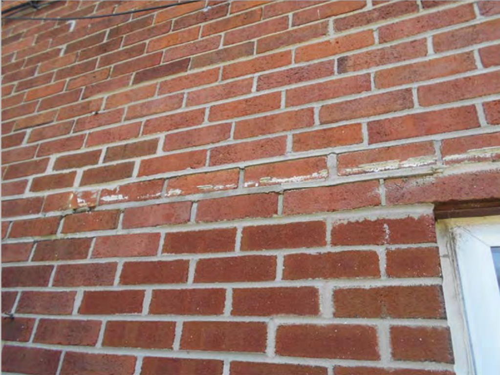
Typical deteriorated brick masonry
