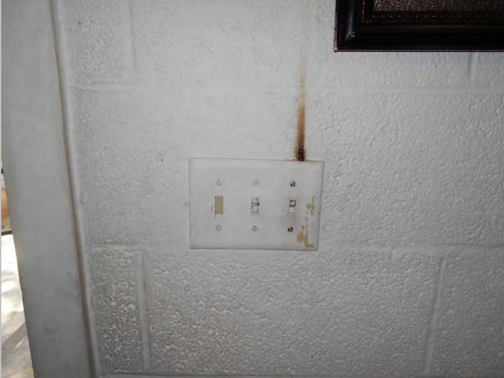
Typical electrical system issues
