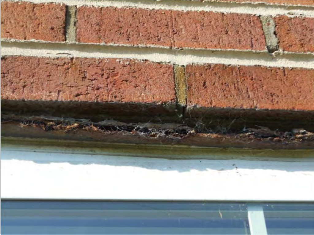
Typical deteriorated steel lintels
