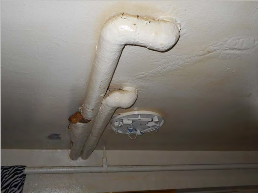
Surface-mounted piping typical in all dwelling units
