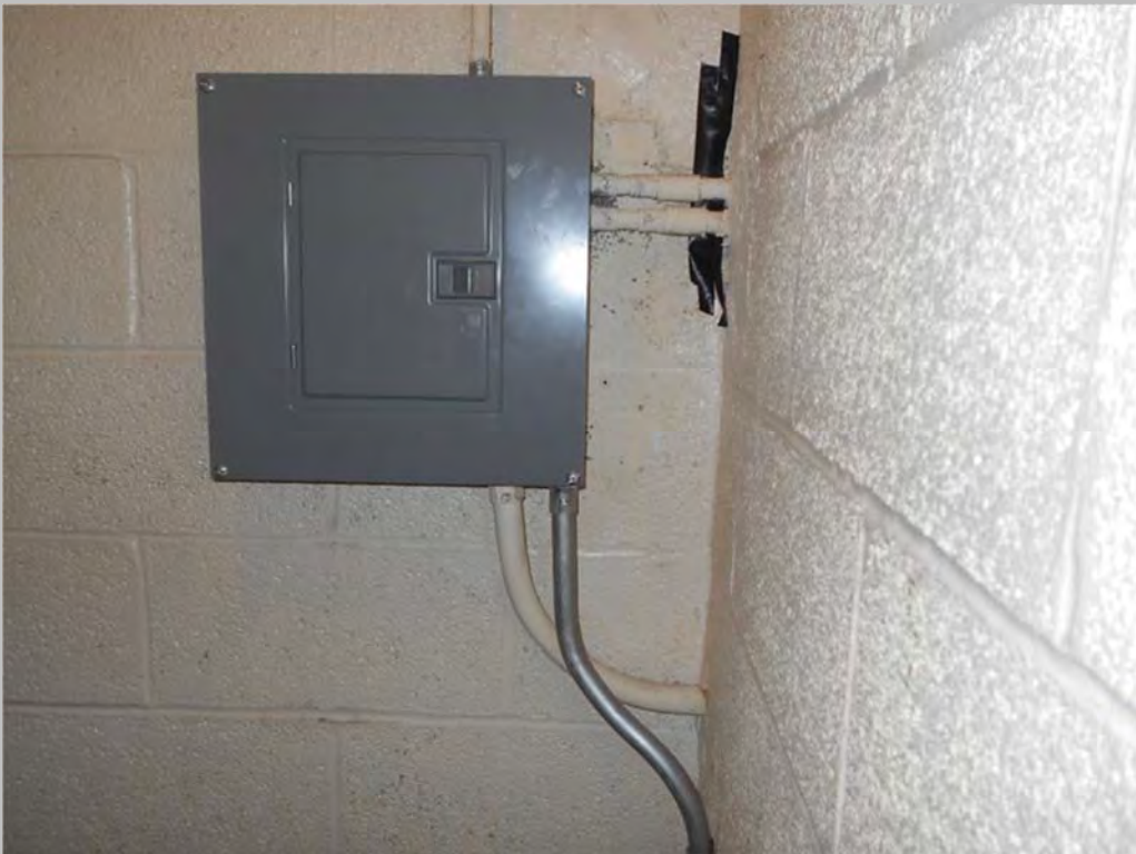
Typical small dwelling unit electrical panel
