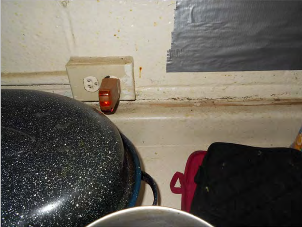
Typical kitchen outlet without GFCI protection
